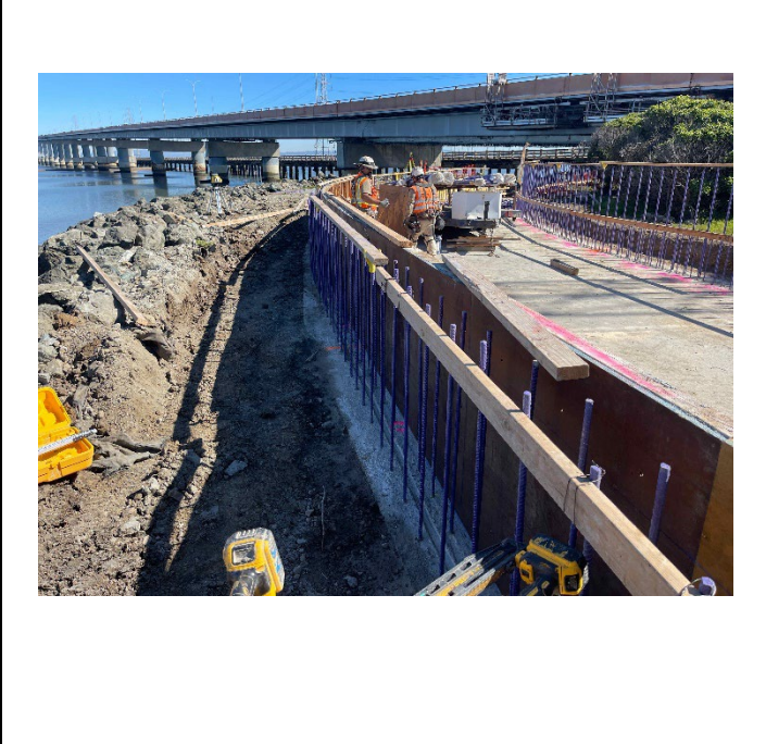
Formwork placement for Floodwall 25 and Floodwall 10 near ~Sta. 98+25 in Phase III (near the SM Bridge)
