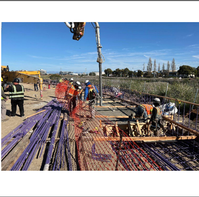
Placement of concrete for the Floodwall 04 footing near Baywinds Park in Phase III
