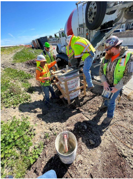
Concrete placement for street light foundations along Beach Park Blvd in Phase II
